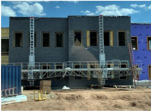
First section of brick veneer is completed on the West end classroom wing (05/31/2022)
