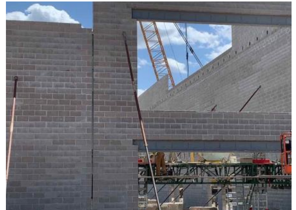
Masonry wall is braced until structural steel is connected at the top (05/16/2022)
